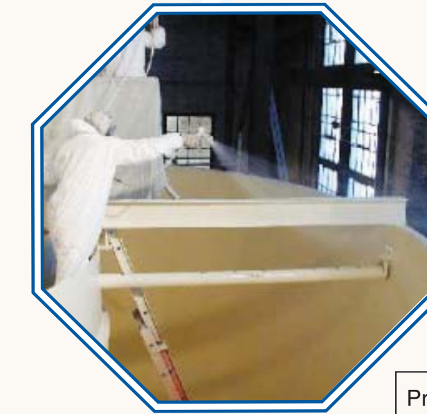
Clarifier Tank USA
